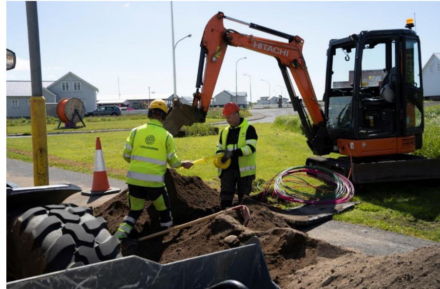
Figure 5: Retractable pipe laid in Ljósleiðari trench in Stokkseyri. Photo: Arna Rut Hjartadóttir
